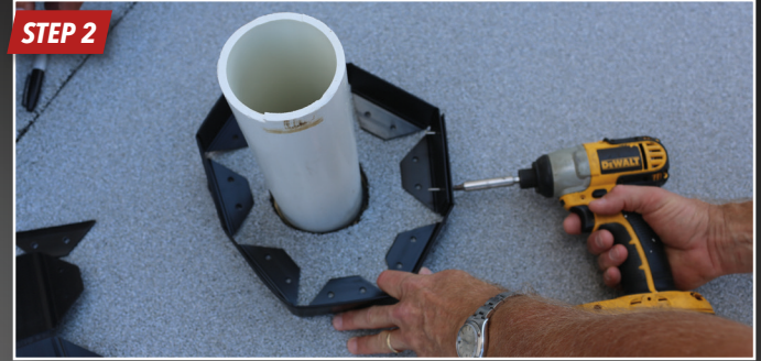
Apply Uniflex MS Hybrid Roofing Sealant in between the two overlapping panels of the fencing and insert a screw to secure the exterior panel foot and two end panels together. Position the fencing around the penetration area and trace around UNIFLEX® Pitch Pan outside wall.
