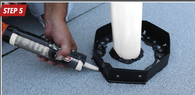
Use Uniflex MS Hybrid Roofing Sealant to seal the perimeter of the pocket where it meets the roof substrate.
